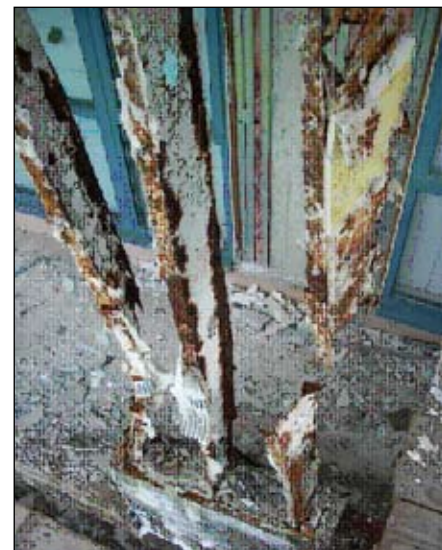
Residential High-Rise Envelope Failure – Steel Stud Corrosion
